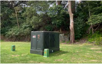
Existing kiosk substation
