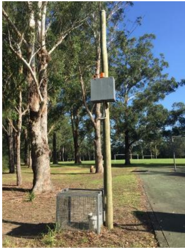
Figure 27. Flood Warning System at Roweena Road, Narara (Historic photo)
