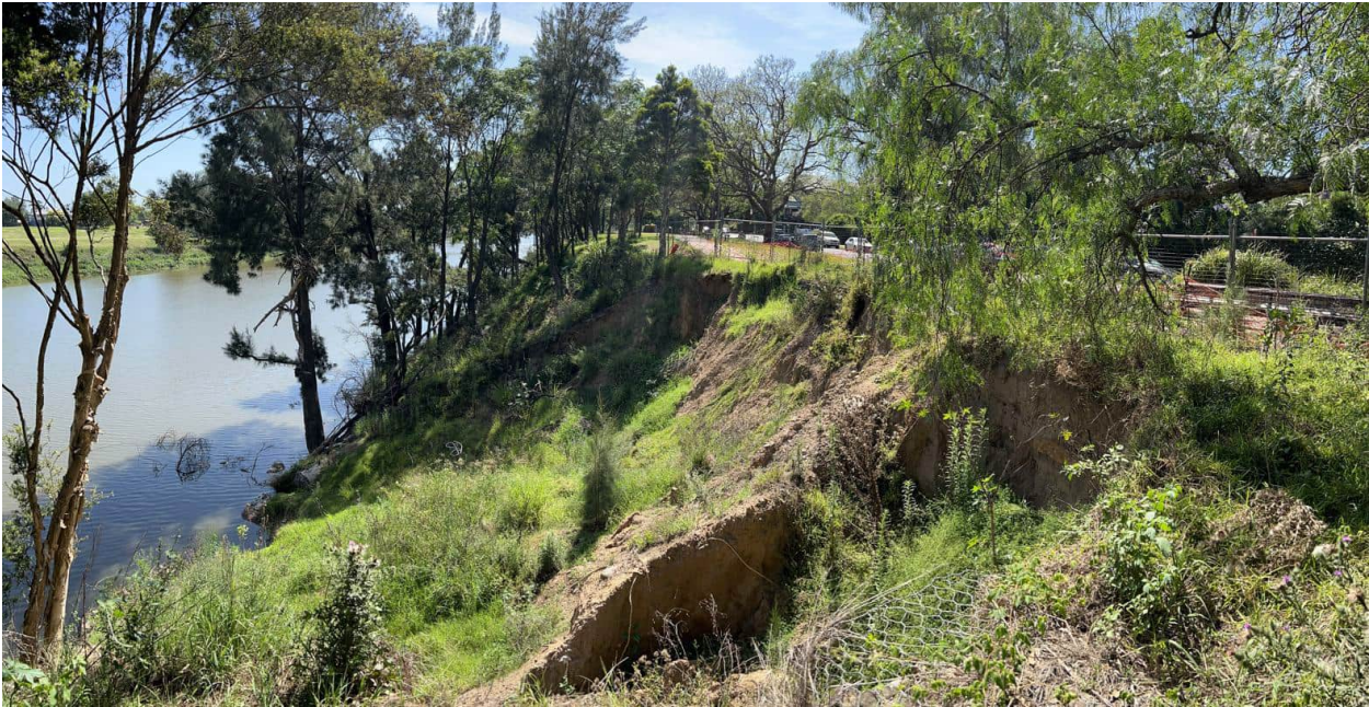
Figure 3-8 Bank erosion at Argyle Bailey Reserve, Windsor
