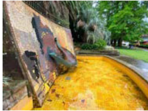
Figure 22: View of the memorial fountain prior to the installation of a steel screen base to prevent public drowning. [Source: Submission by Merril Jackson to public exhibition of the draft Burns Place CMP]
